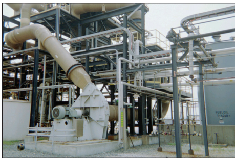
The induced draft fan is shown in the above photograph.
