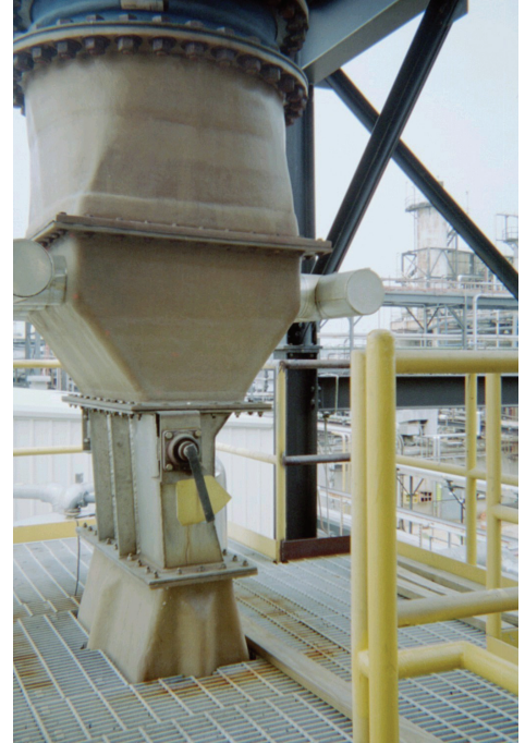
Above is shown the feed duct with the venturi upper section with an adjustable throat.
