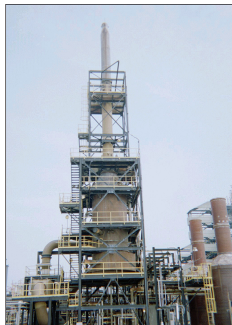
Above is the venturi and chevron separator assembly. The stack in the middle is the old WESP.
